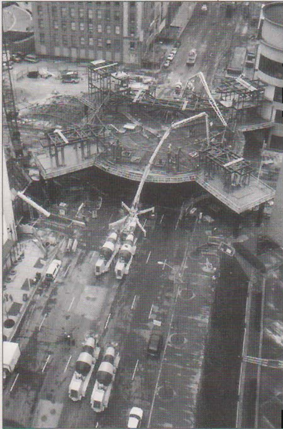
R. L. McCoy's pair of Schwing concrete pumps receive plasticized mix from dual Carmel Concrete ready-mix trucks and place it on deck of the Artsgarden at Indianapolis' Washington and Illinois streets intersection.
