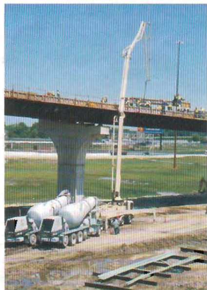
Placing concrete for a nine-span, 1,140-foot-4-inch flyover ramp from eastbound I-74 to southbound I-465.
